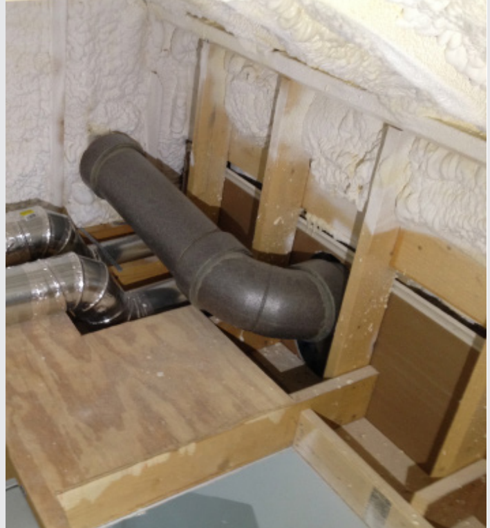
ComfoPipe duct routed to exterior grill
